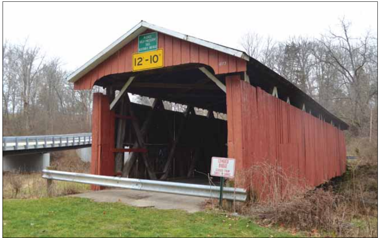
Restoration on the covered bridge near Stevenson Road is expected to begin in the spring.
